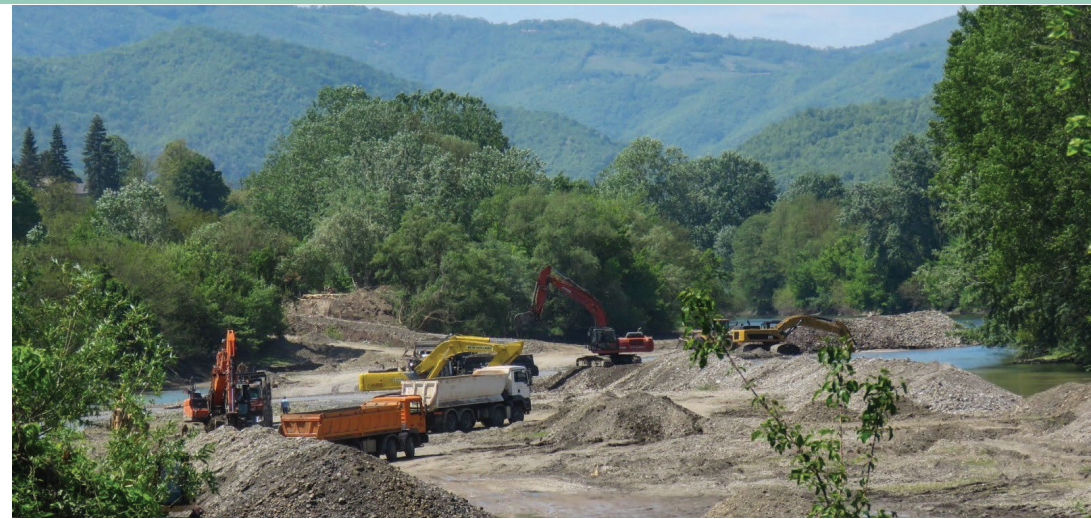
Image 2: Illegal excavation of gravel in Western Morava (source: www.pakt.org.rs)
